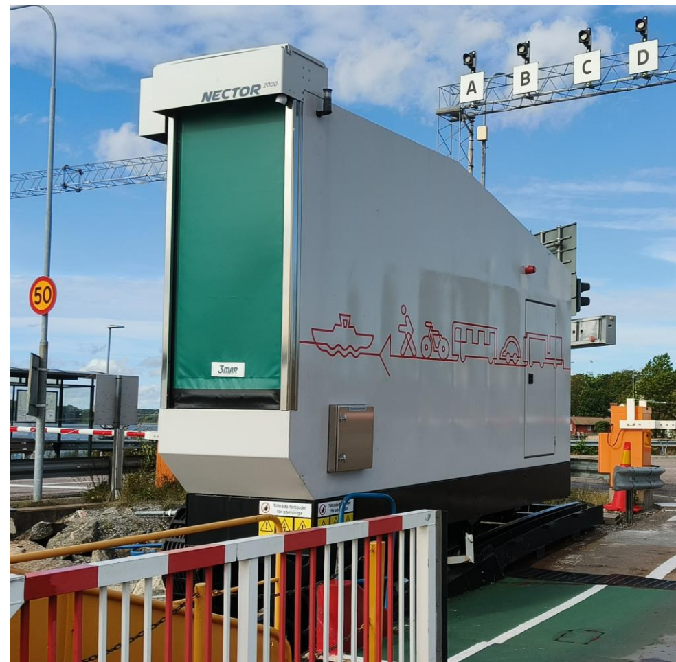
Nector 2000 Charging connection device in Vaxholm, Sweden.
